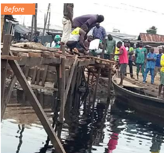
A bridge construction work-in-progress by iLEAD students from Fazil Omar Senior High School
